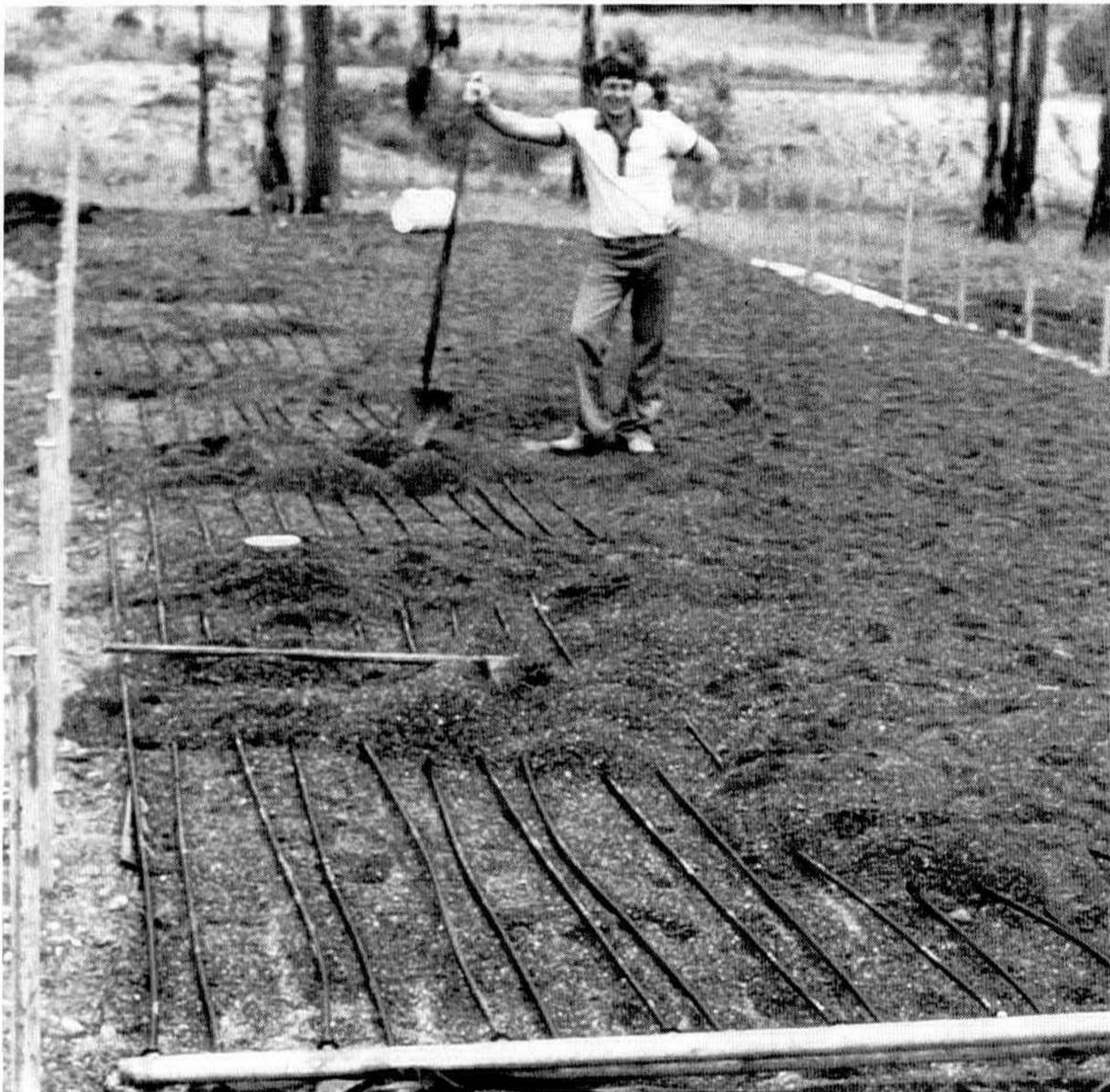
Figure 4. Heat lines are laid in a sand bed then covered with matting.
